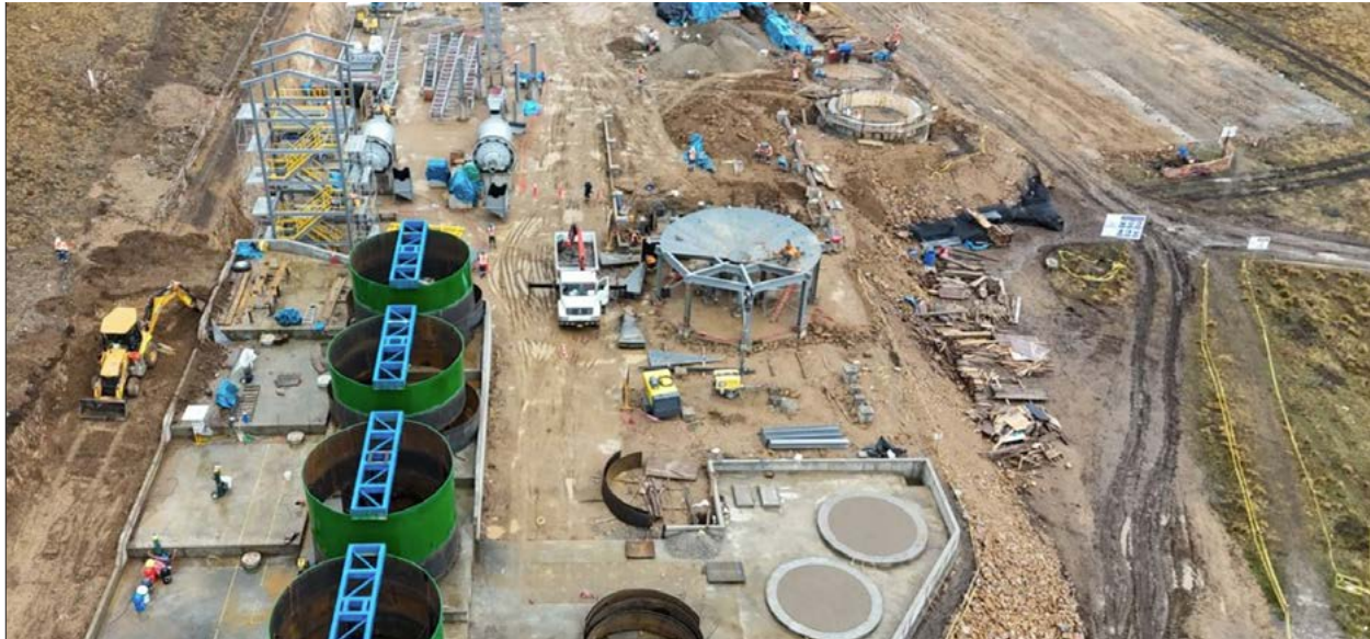
Construction of the beneficiation plant at the Igor project in Peru. Source: PPX Mining Corp. website
